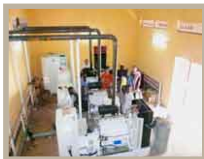
The power plant at Garalo runs on Jatropha oil
