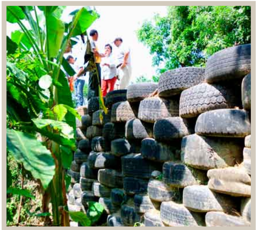
Contention wall demonstration project, built according to the community's own initiative using recycled tyres to stabilise the slope in San Bernardo Guatemala
