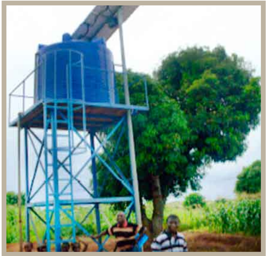
Photovoltaic panel and tank for Mzee Disaster Risk Reduction Club
