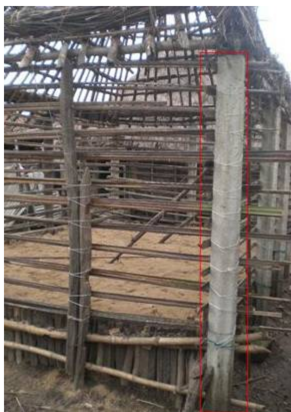
Photo 5: Reinforced concrete pylons made with cement and sand now take the place of stilts (Afintin trunks)
