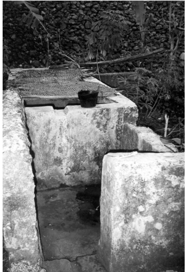
Open reservoir with loose cover and bathroom with drainage
